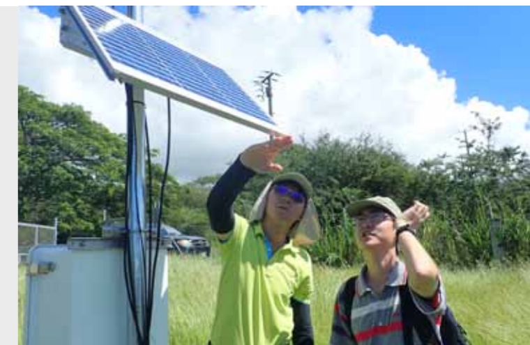
Project technician Sung-Han You (left) and Central Weather Bureau expert Shao-Liang Sung (right) consult on the installation of meteorological station equipment.
